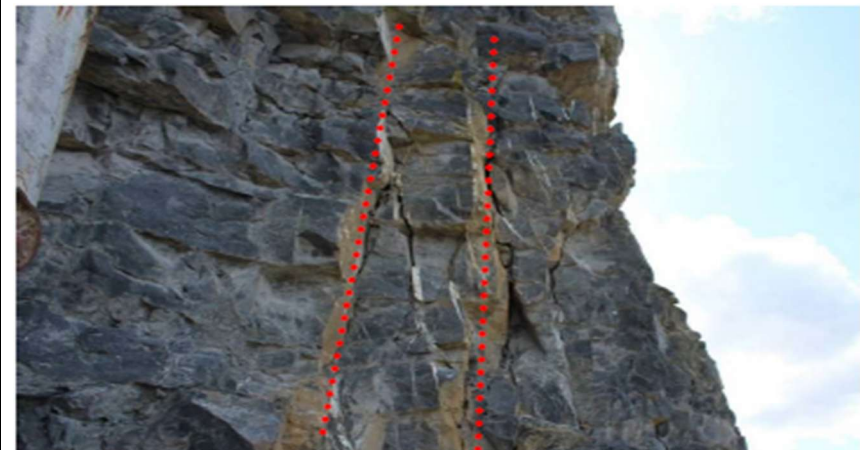
7.1(d) The secondary joint set in a boundary wall with the application area.
